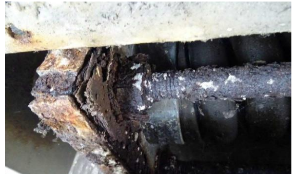
Gallows Corner Flyover (steel fatigue) Daily users – 38,000
