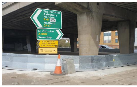
Brent Cross Structures (all over structural condition – very poor, temporary parapets in place) Daily users – 175,000
