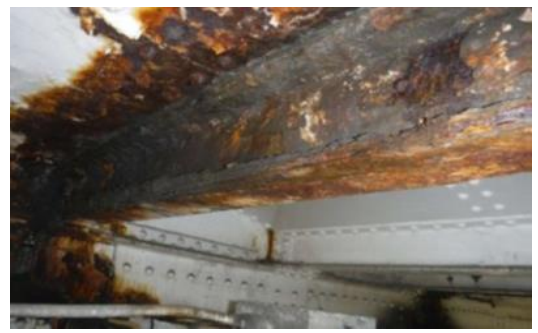
Vauxhall Bridge (steel fatigue / overall condition – very poor) Daily users – 47,000
